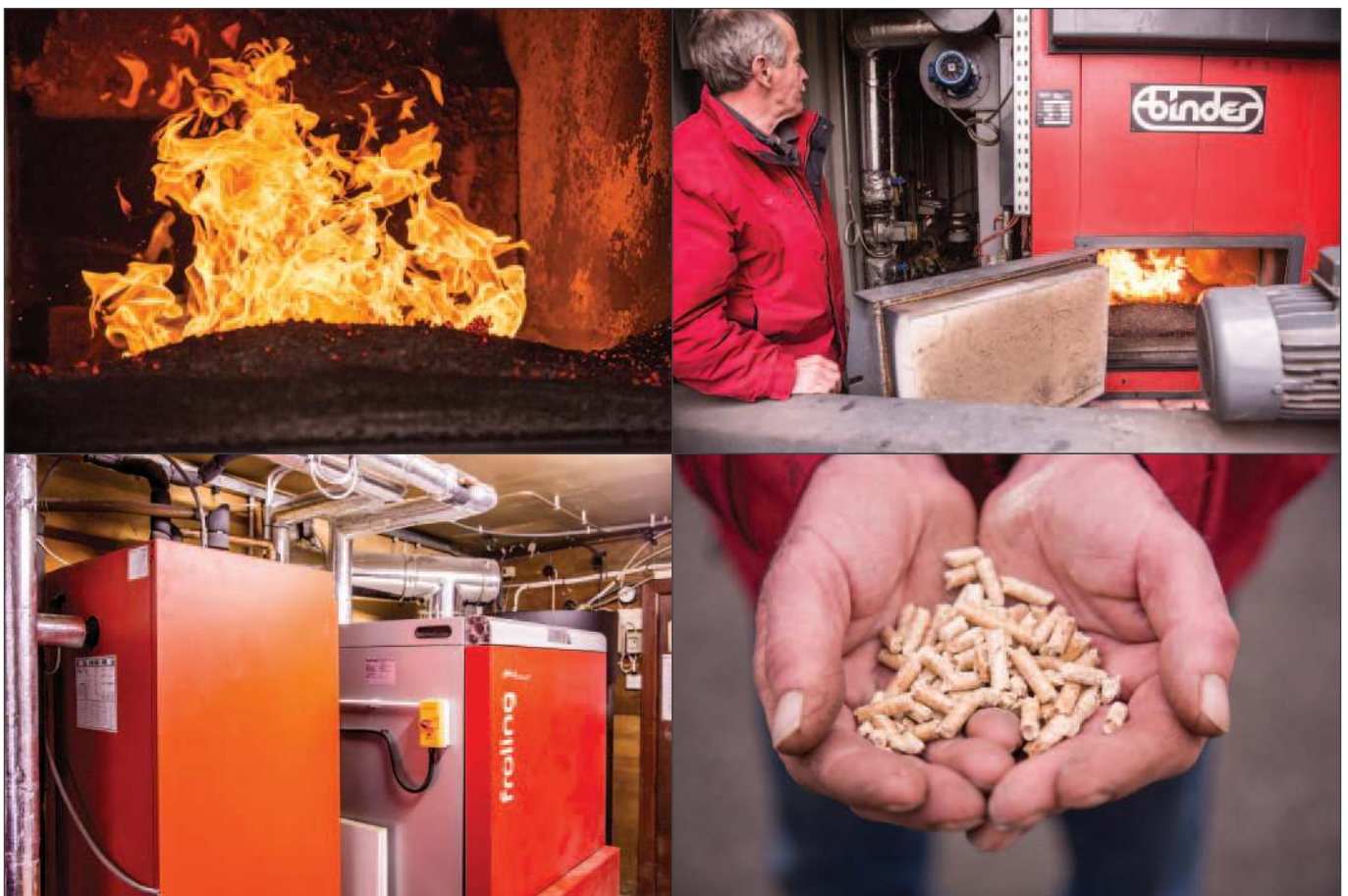
Pictured: Wood Pellet Biomass System, Manor House Hotel, Enniskillen and Valley Hotel, Fivemiletown
